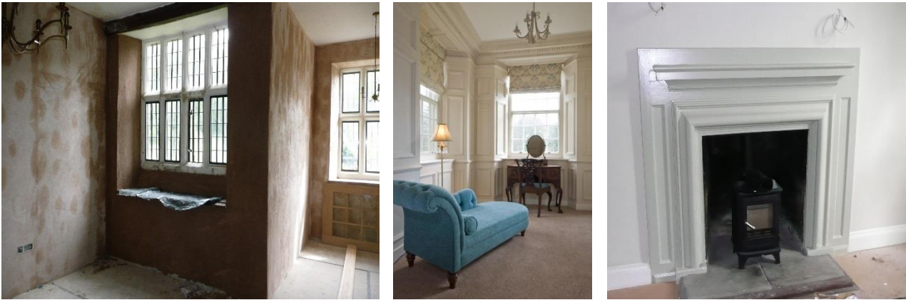
From left: Window repairs plastering, joinery and glazing. Resulting in simple, stylist and comfortable accommodation.
