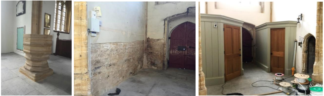
(left) The font re-situated on a plinth and new portland flooring, (middle) after the removal of the church organ, (right) the installation of toilets.
