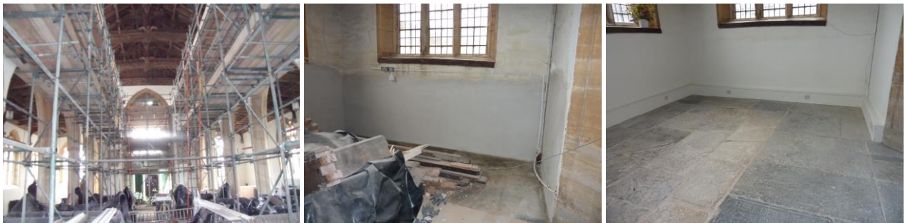
Scaffolding up to the clerestory windows enabling render and masonry repairs. Middle (during) and right (after) render repair and new flooring.
