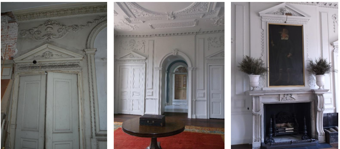
From left: Plasterwork that could be saved was restored throughout. In the White Room, a clean and effortless link is made to the new apartment and Loggia. The fireplace was reinstalled. New decorative stonework and joinery repairs frame the portrait blending with surrounding plasterwork and panelling.
