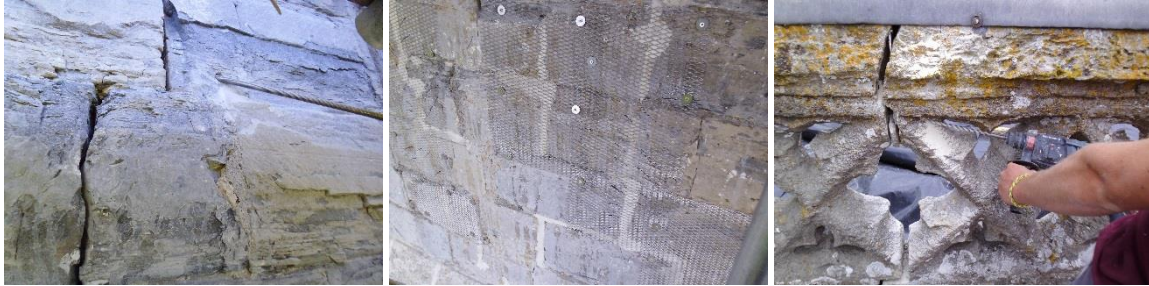
Repairs in progress showing removal of poor historic repairs and securing repointed stonework with steel mesh.
