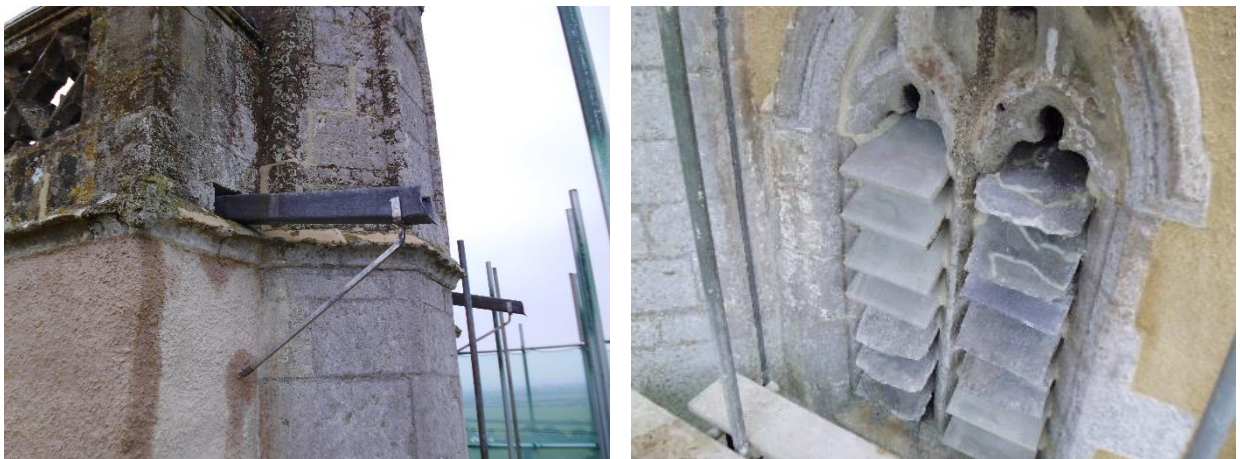
Specially commissioned lead shutes in place supported by steel fixings, and new belfry louvres blend with originals.
